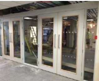
Image courtesy of Prestige Fire Door Services
